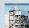
Combustion plants for the disposal of exhaust air, waste gases and liquid media
