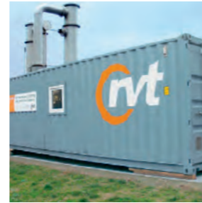
RVT's multi-purpose plant
