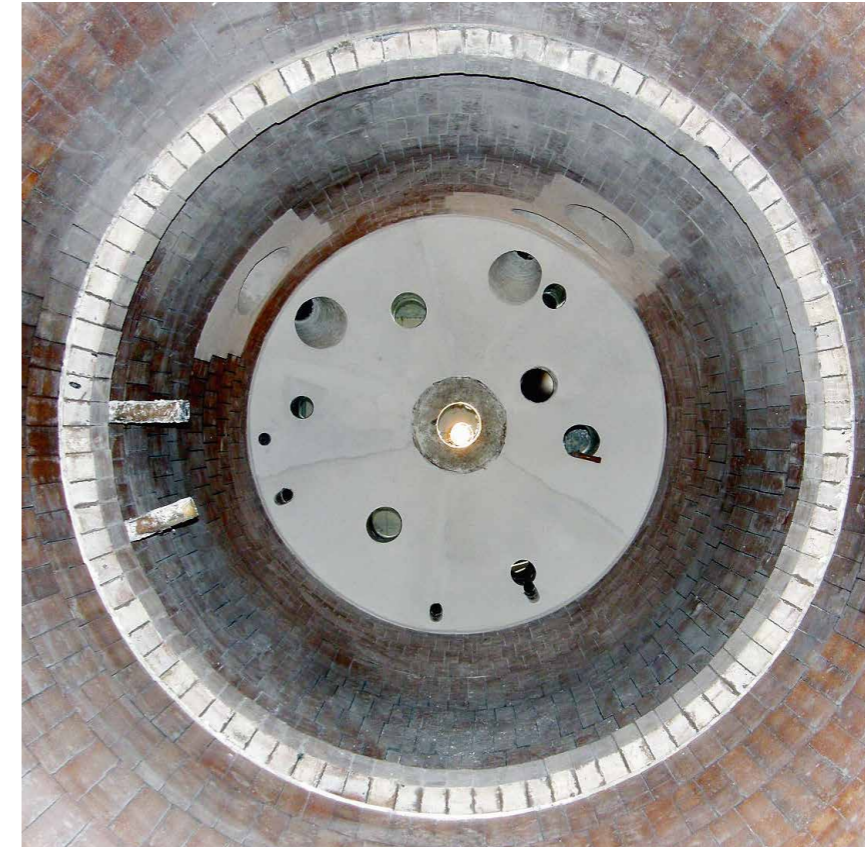
Refractory lined combustion chamber
