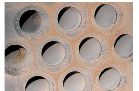
Gas tube boiler for waste heat recovery
