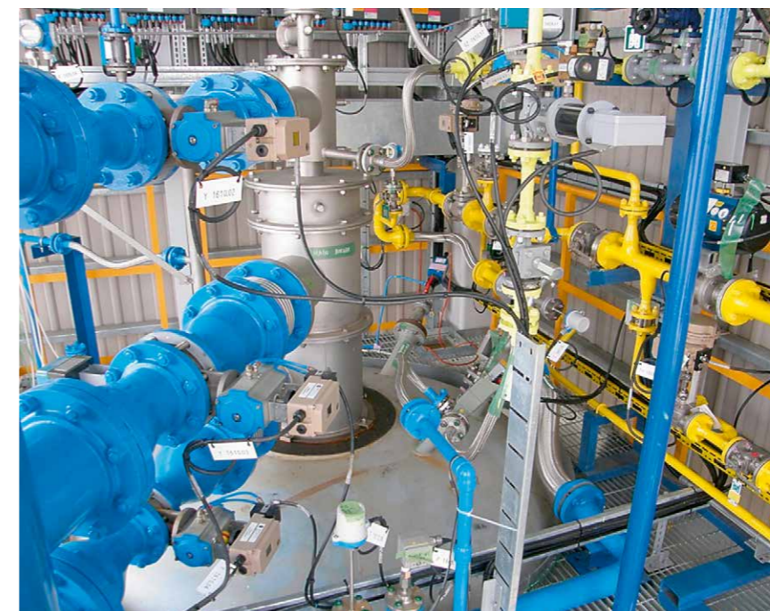
Burner with fuel and waste gas piping
