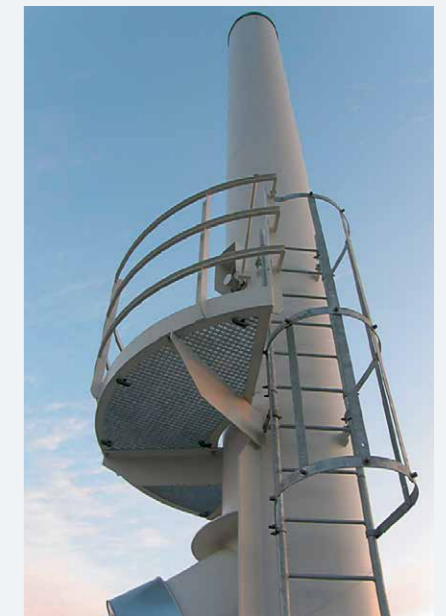
Flue gas stack with emission control device
