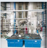
Ammonia recovery processes
